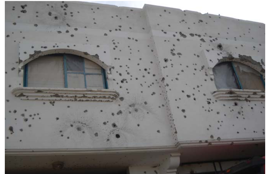
Damaged Exterior Wall in Gaza City | UUSC
