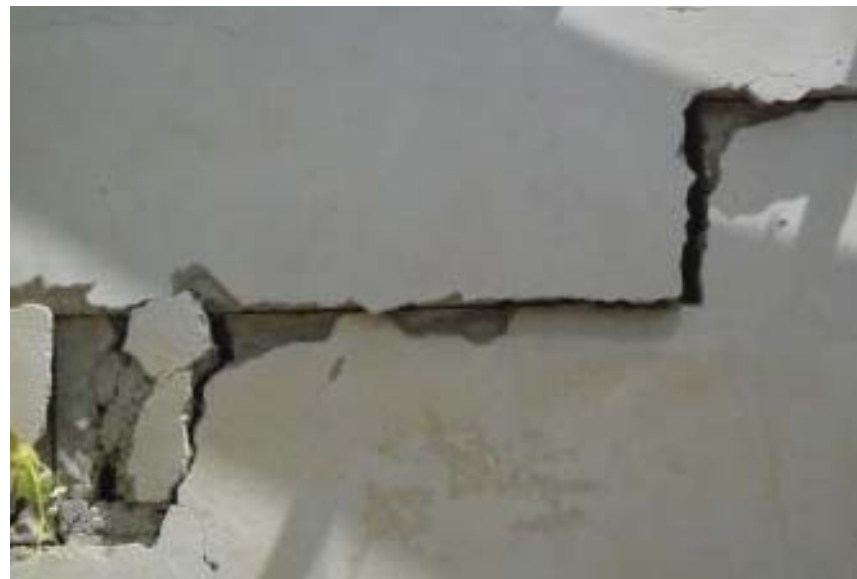
Cracking Wall in Gaza City | UUSC
