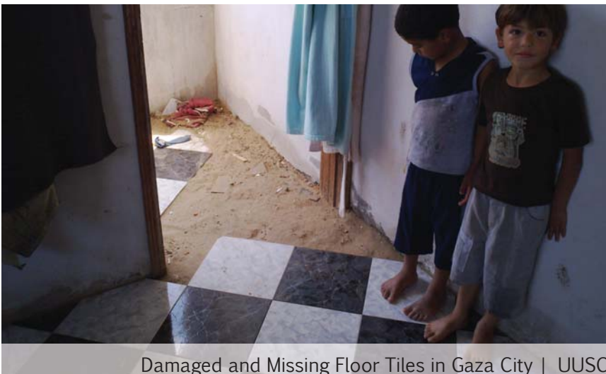
Damaged Bathroom in Gaza City | UUSC
