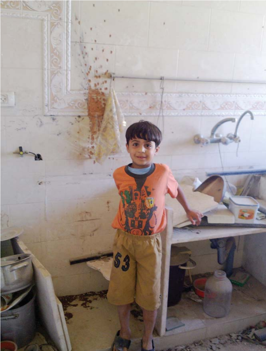
Damaged Kitchen in Gaza City | UUSC
