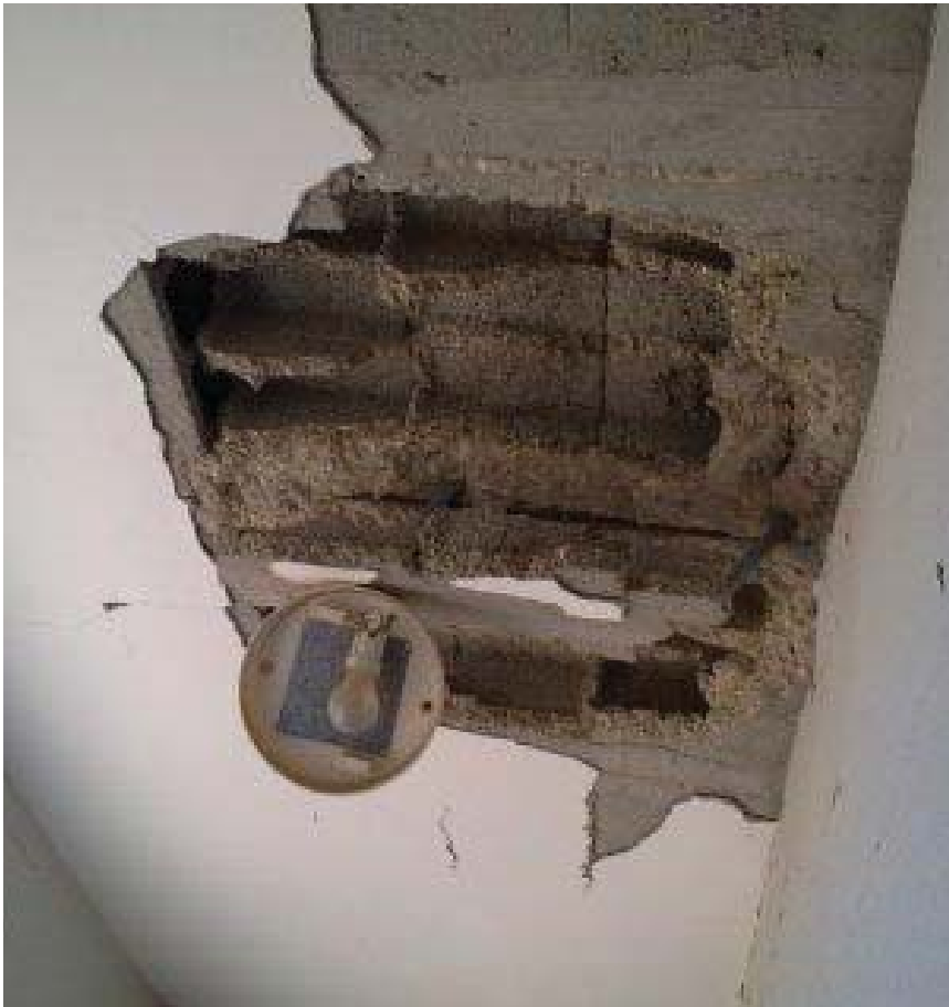
Interior Plaster Damage | UUSC
