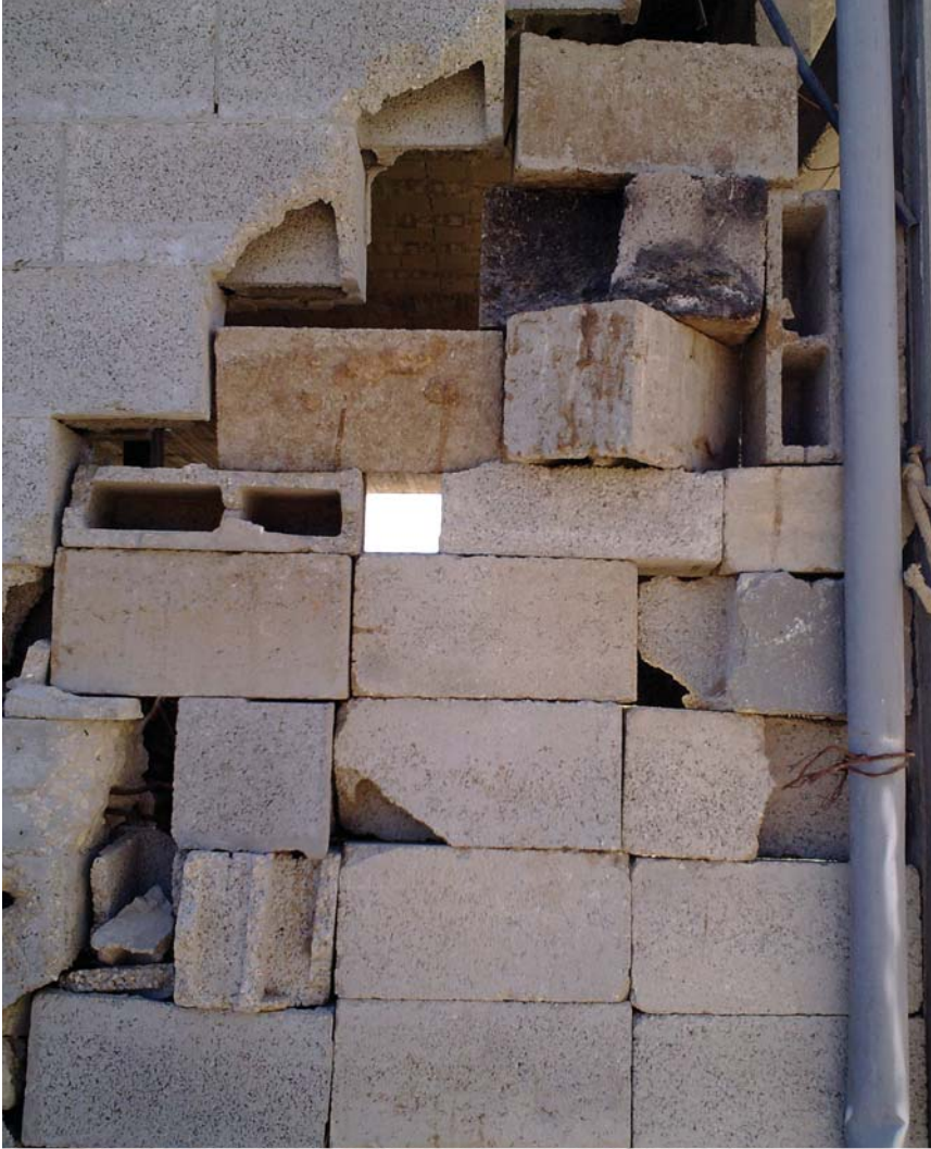
Structural Damage in Gaza City | UUSC
