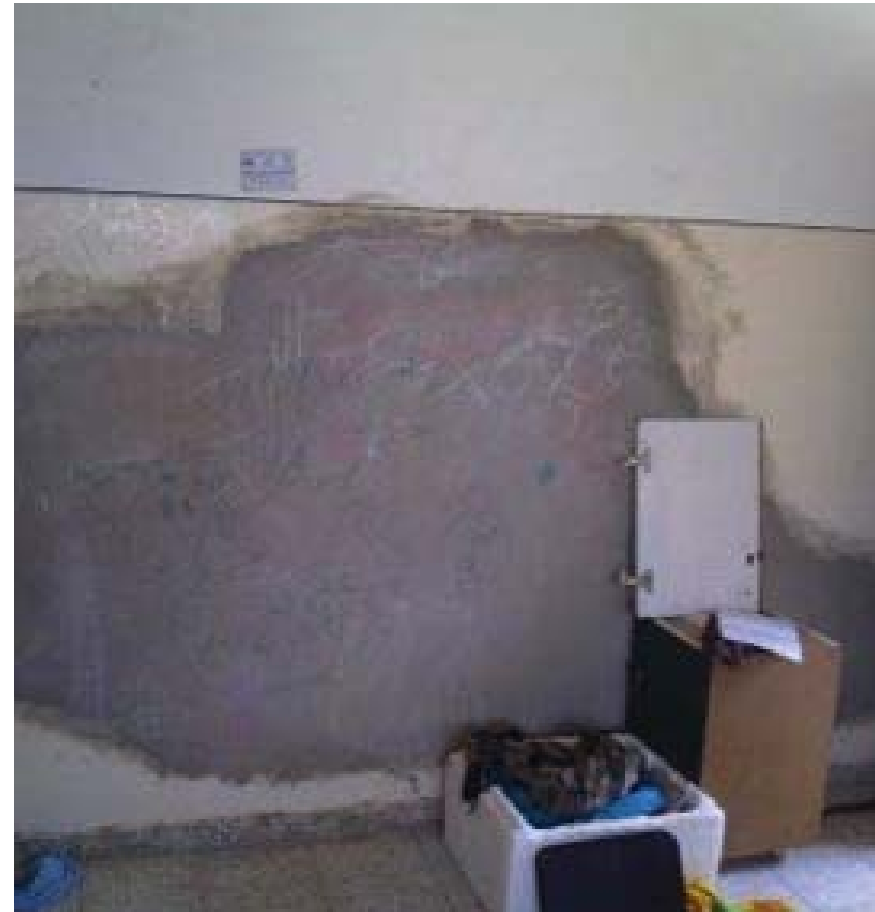
Interior Painting Damage | UUSC
